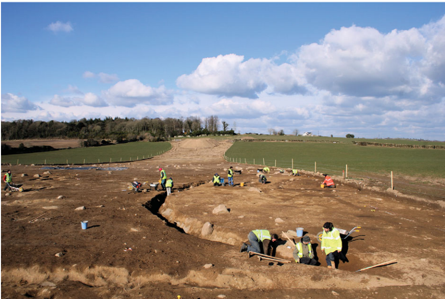
A pair of photographs taken on the N9/N10 Kilcullen to Waterford Road Scheme demonstrates the ongoing relationship between road construction and archaeology in Ireland. Top: an excavated section of a slip road in the Townland of Ballybannon shows part of an Iron Age ringfort; the remainder of the ditch is clearly visible as a crop mark in the ripening wheat to the left of the photograph. Bottom: a multi-period site located 10km to the north-east in the Townland of Russelstown was excavated within the main road corridor and included the remains of an Early Neolithic building, Final Neolithic/Early Bronze Age features, a medieval enclosure, archaeometallurgical activity, and post-medieval ditches and features. Both excavations were undertaken on behalf of Kildare and Carlow County Councils and the National Roads Authority by Headland Archaeology (Ireland) Ltd whose collaborator, Brian MacDombnaill, submitted the images.
