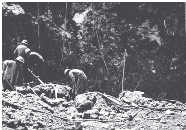
Fig. 1. Excavation of material for the construction of the Grande Dixence dam in ice-rich permafrost of a rock glacier at the locality Prafleuri, Valais Alps, Switzerland. (Photo: W. Fisch 1956; cf. Fisch and others, 1978.)
