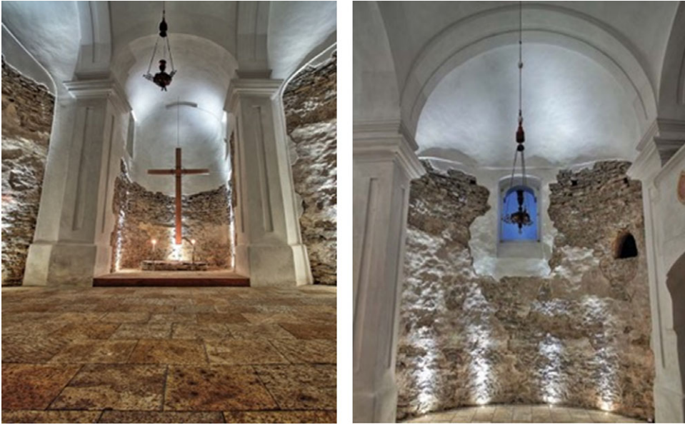
Figure 3 Interior view of the Rotunda (left) and the nave's southern wall with the original pre-Romanesque window opening after the restoration (right).
