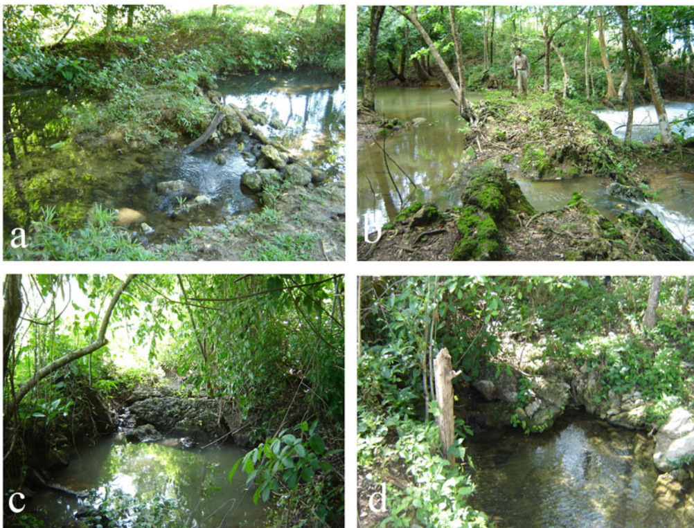
Figure 7. (a–d) Examples of abutments/bridge foundations recorded in the study region (image by author). (Color online)
