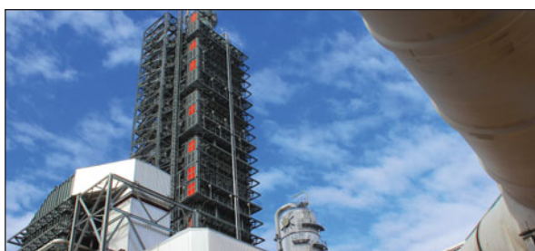
A 16-foot-diameter duct takes flue gas from a coal plant at the W.A. Parish generating station near Houston, Texas, to the Petra Nova carbon capture facility. There, carbon dioxide is removed by an amine solution in the tall absorption tower; separated from the amine as 99.9% pure carbon dioxide in the smaller regenerator tower to the right; and then compressed and delivered to an oil field. Photo: Business Wire .
