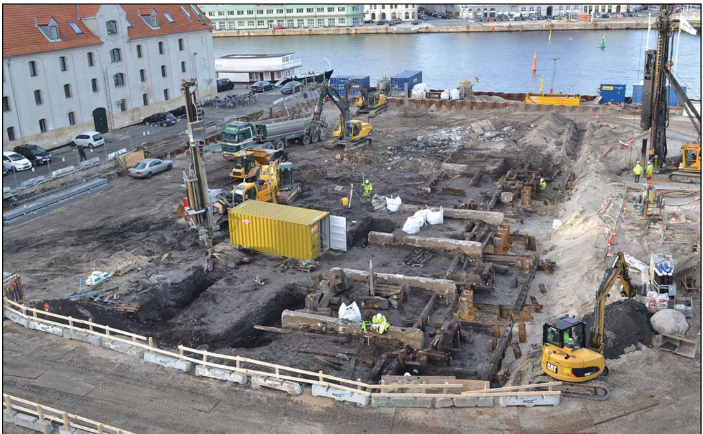
Figure 2. Excavation at Krøyers Plads in the centre of Copenhagen, Denmark (photograph courtesy of the Museum of Copenhagen).
