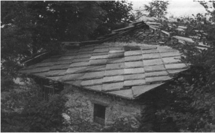
Roof in the antique and rustic manner, squared slabs of split gneiss from the quarries of the Luserna valley, re-made 1992 by the master-roofer Rinaldo Jourdan on a restored upland baita, at altitude about 1100 m, near Torre Pellice.
