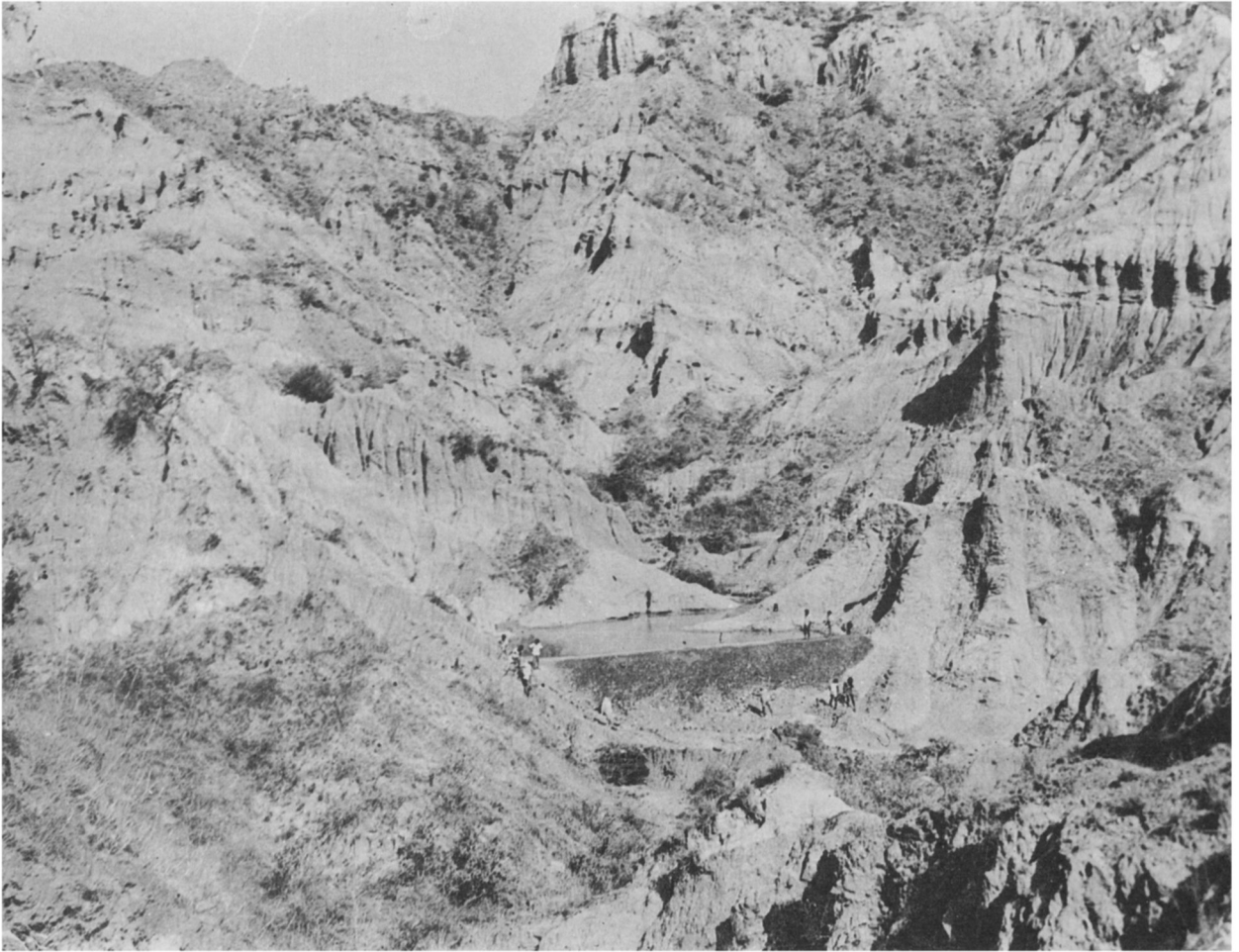
FIG. 1. Denuded hills of Sukhomajri and, in centre, construction of a check-dam in progress. Human figures on the dam indicate the scale.
