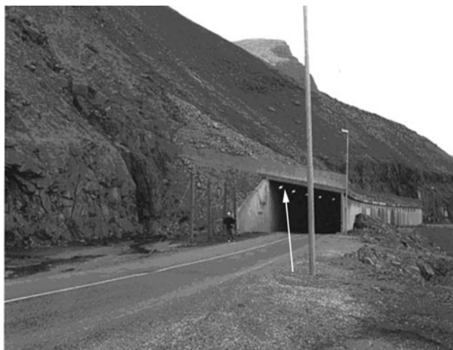
Fig. 6. Concrete shed and location of sensors on the inside hillside wall in path 15.
