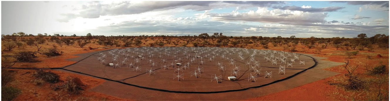
Figure 4. A panorama of the EDA looking north. In-field beamformers (small white boxes) each service 16 dipole antennas. The thick black cables are the 200 m coaxial cables running between the beamformers and the shielded room.
