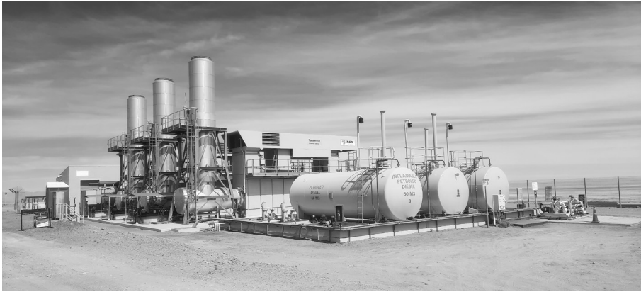
Figure 9.2 The ALMA power plant built by TSK Elektronika y Electricidad S.A. The plant uses Taurus 60 gas turbine generators, by Solar Turbines. The three 60,000 L fuel tanks on the right side of the photograph store diesel fuel; an additional three tanks, not visible, store 200,000 L each of LPG, enough to run ALMA for three days. Credit: ALMA/ESO/AUI/NINS, CC BY 4.0.
