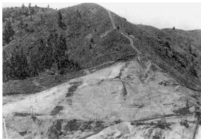
FIGURE 26. Landslide in granite containing abundant zones and seams of beidellite, Anderson Ranch Dam site, Idaho.
