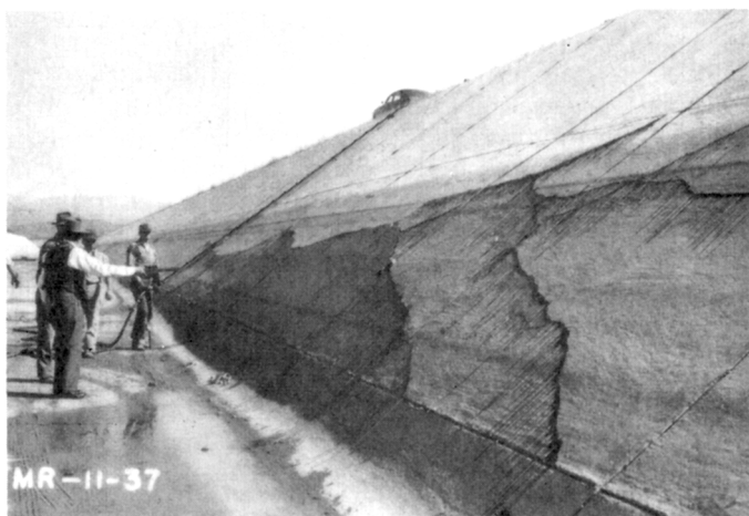
FIGURE 38. Cracking and bulging of concrete lining by swelling of beidellite clay in the subgrade. Friant-Kern Canal, near Lindsay, California.
