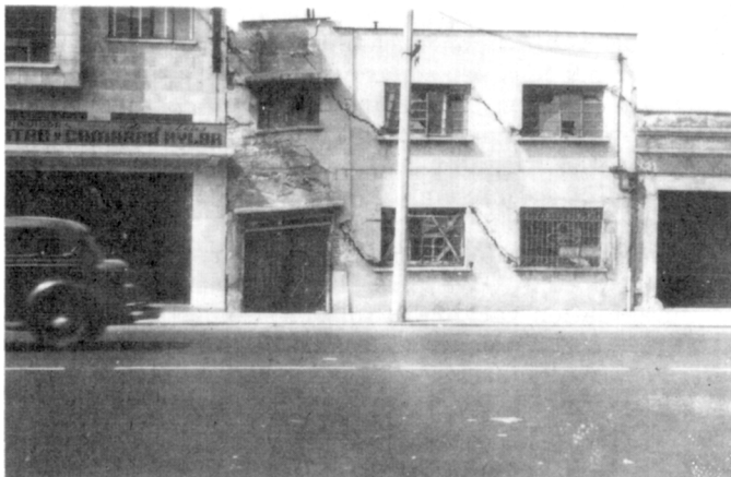
FIGURE 33. Settlement of a building as the result of consolidation of montmorillonite clays in the foundation, Mexico City, Mexico. Courtesy of A. E. Cummings (1947).
