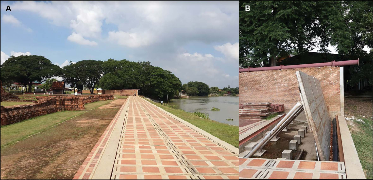
Figure 3. Flood wall disguised as walkway (A) and activated flood defence (B) at Wat Chaiwatthanaram in 2015 (photographs by W. Pittungnapoo).
