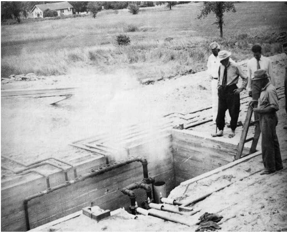
3 Wright testing the floor heating system of Jacobs House I, photographed by Katherine Jacobs. Art Institute of Chicago, Herbert and Katherine Jacobs Residence and Frank Lloyd Wright Records, Ryerson and Burnham Art and Architecture Archives, digital file #197701_220408-023.
