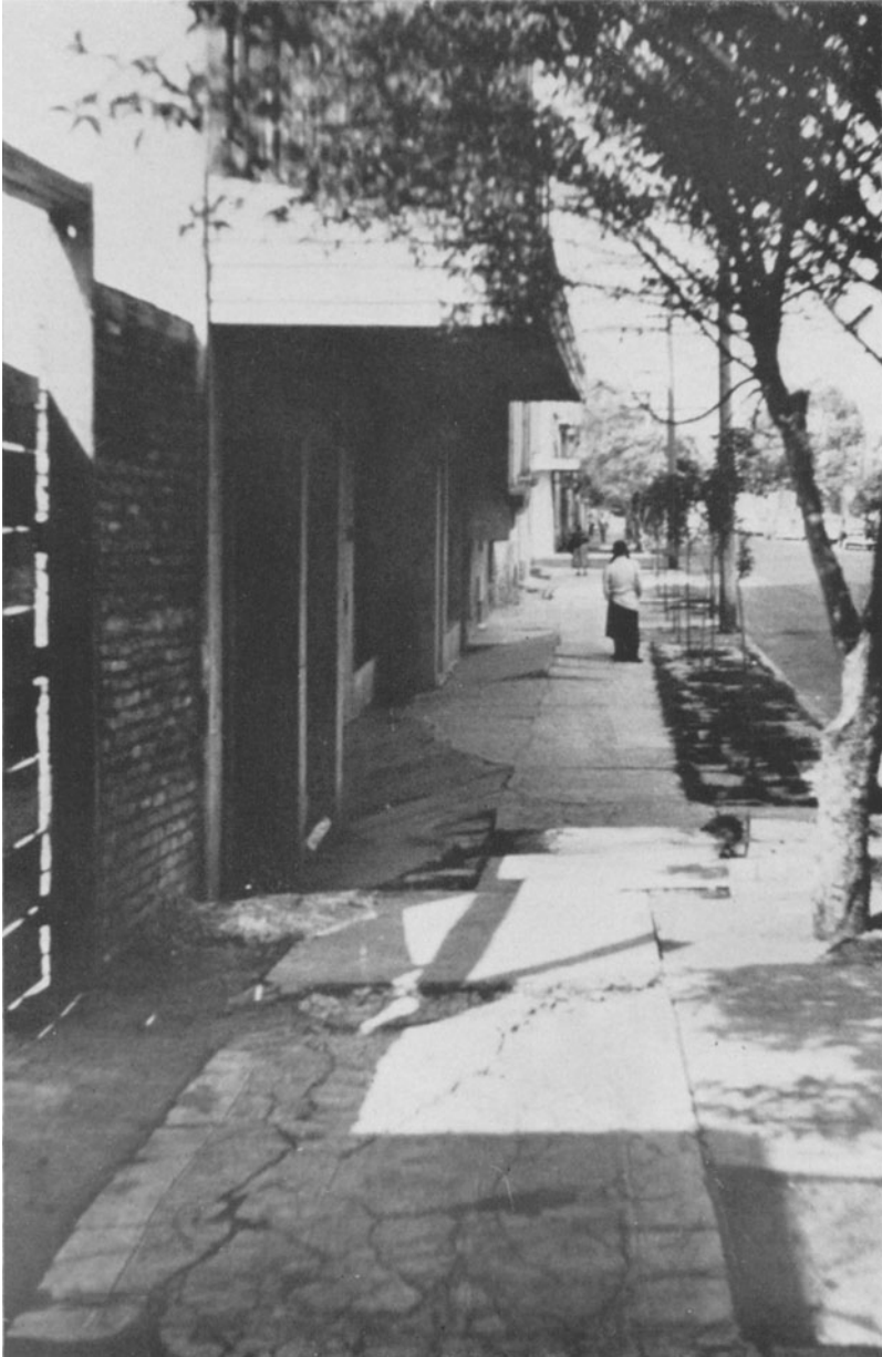
PLATE 2.—Settlement phenomenon, still an unsolved fundamental problem.
