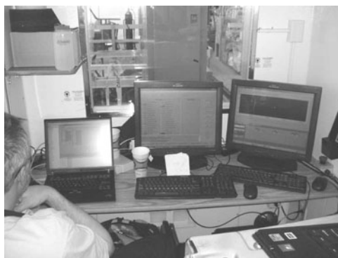
Fig. 10. Inside of control room.
