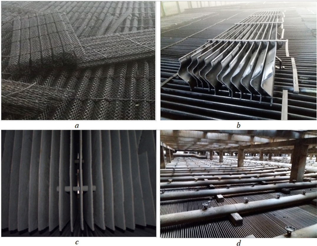
Figure 4. Photos of ORS RNPP cooling tower elements for 2022 (a, b—condition of water traps; c, d—condition of sprinklers).
