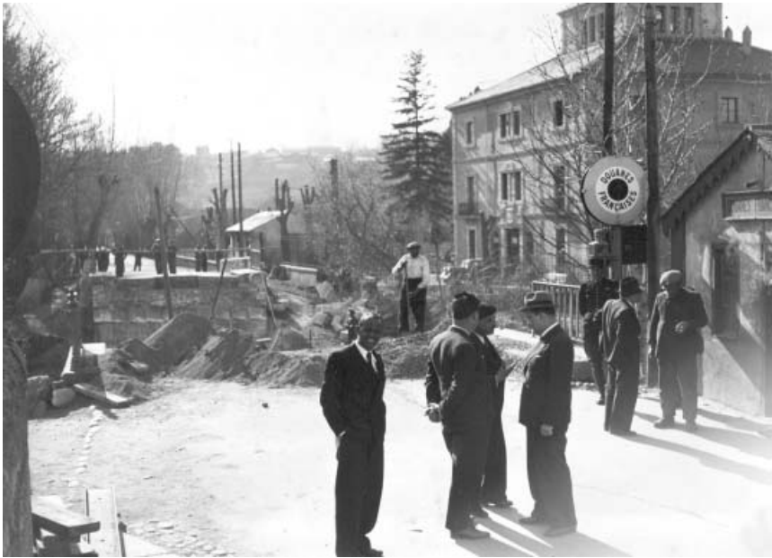
Figure 4. Broken-up road at border crossing in Bourg-Madame, 1939. Refugees were forced to cross the French–Spanish border through a ford in the nearby river.
