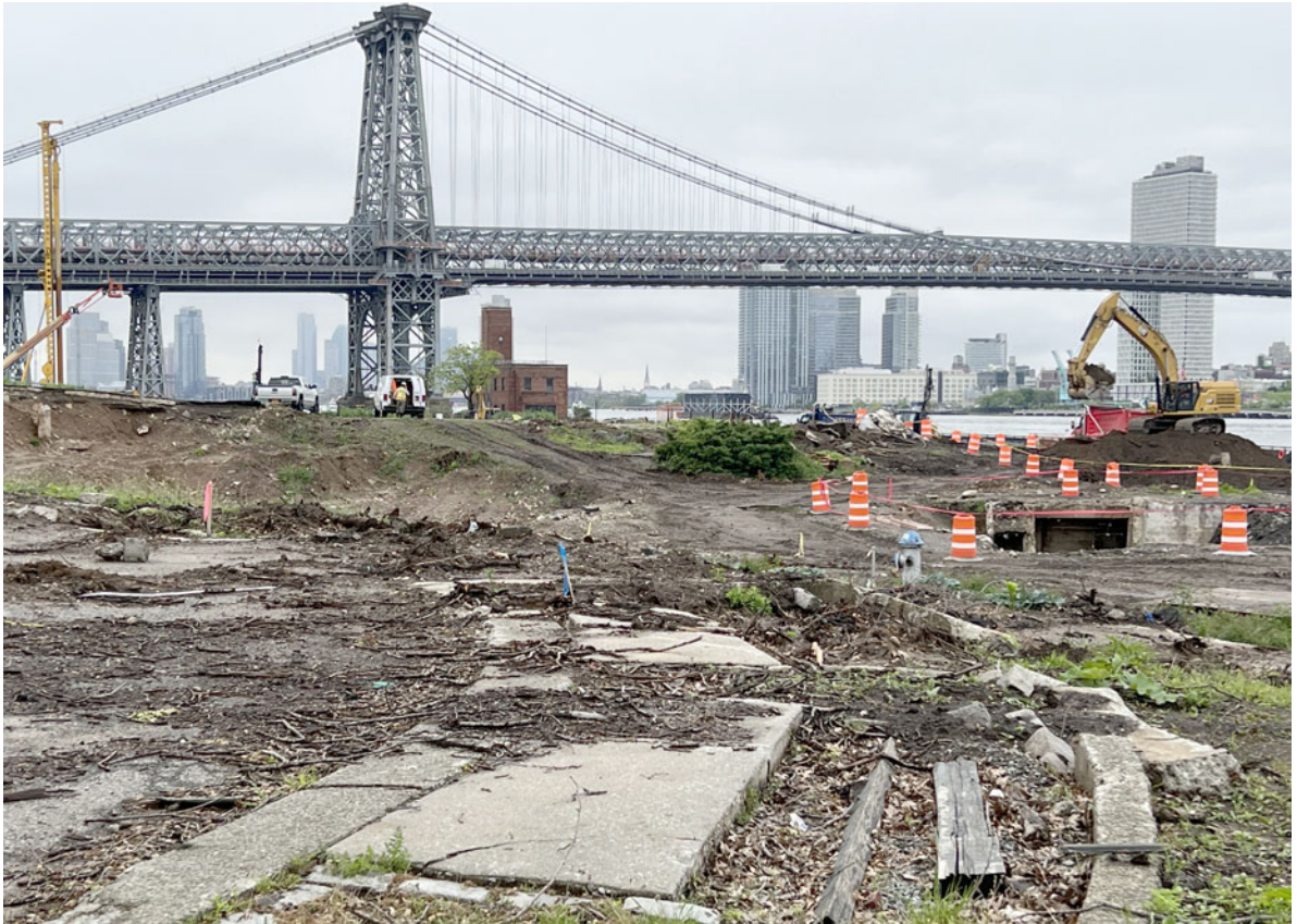
FIG. 2. Demolition of the southern end of East River Park. Photo taken by the author, 19 May 2022.
