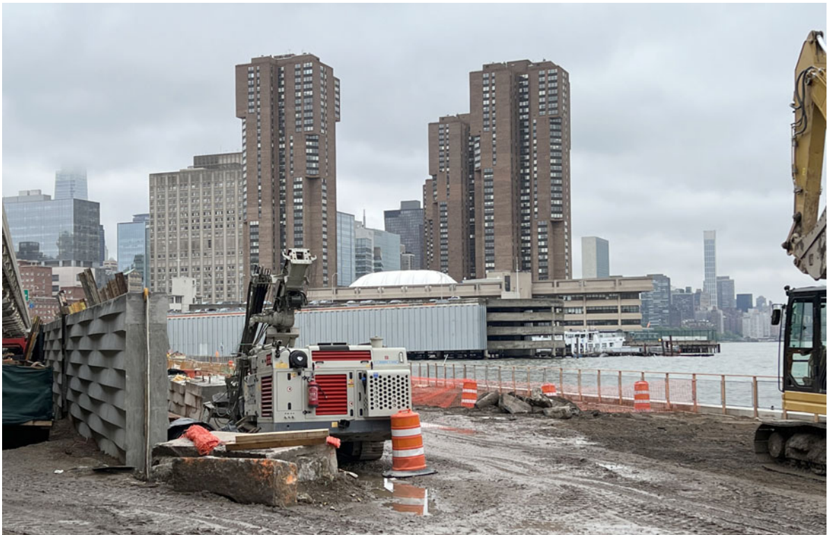
FIG. 4. Installation of the East River seawall near Stuyvesant Cove Park. Photo taken by the author, 19 May 2022.
